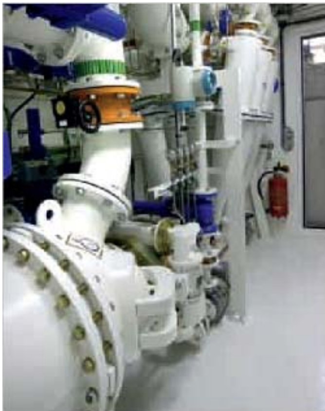
Fine Filter and Cyclones
