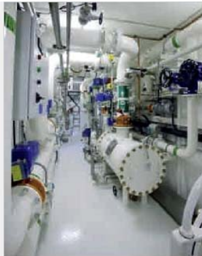
2 x 250 m 3 /h containerized
