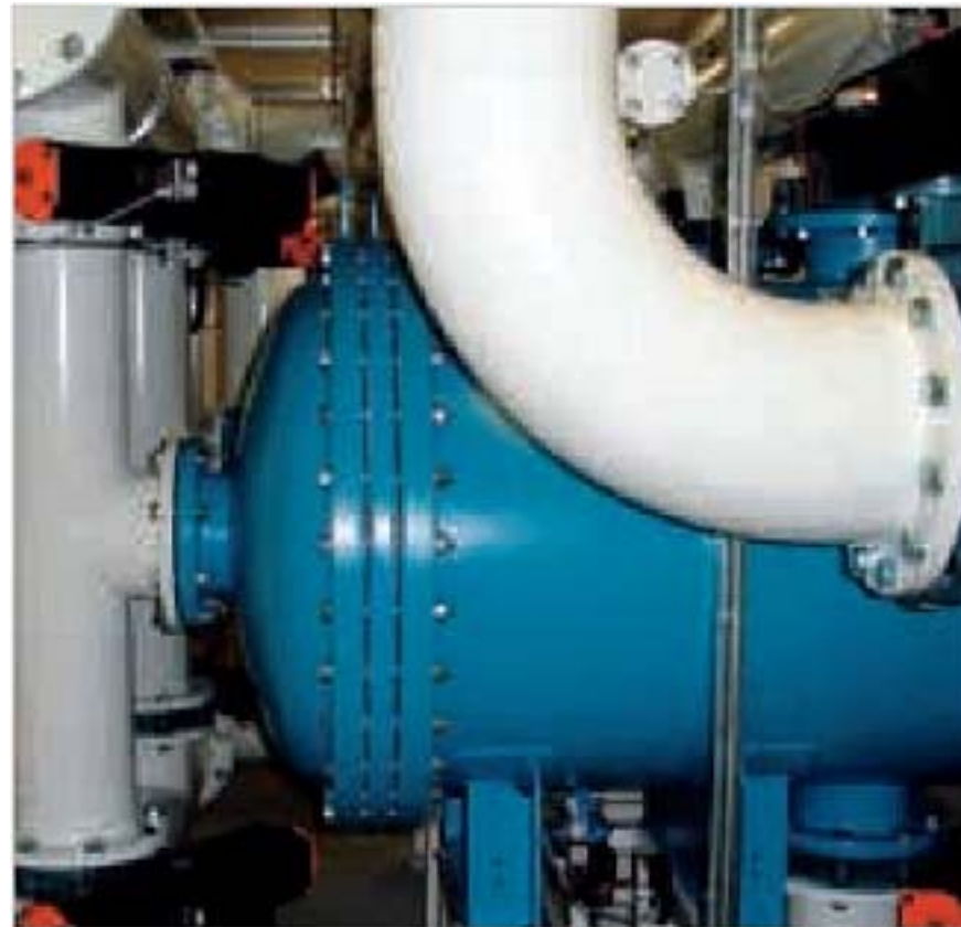
RWO's new ballast water disc filter
